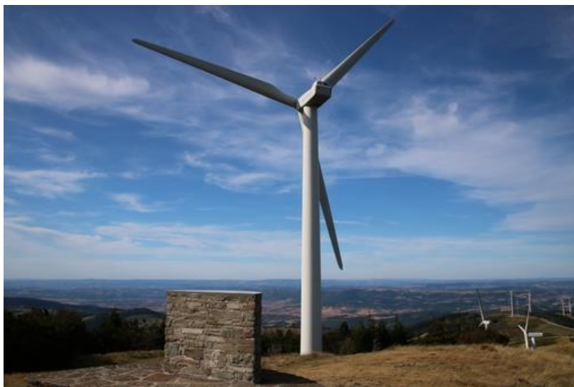
Figura 148. Aerogenerador Nordex N60/1300. Tomado de: (The Wind Power, 2022) .
